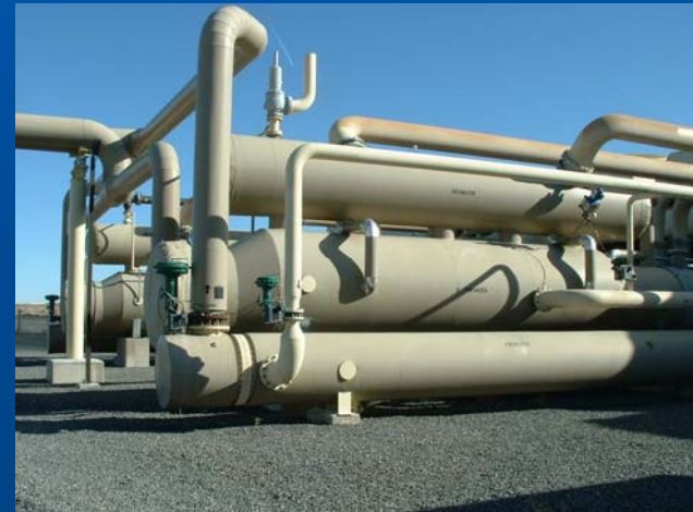
Galena – Geothermal plant
