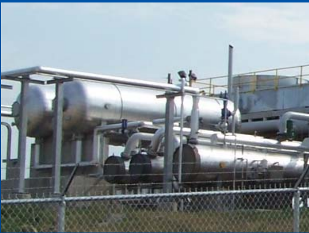
Heat Exchangers – preheater and vaporizer set
