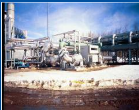
Heat Recovery - Pipelines
